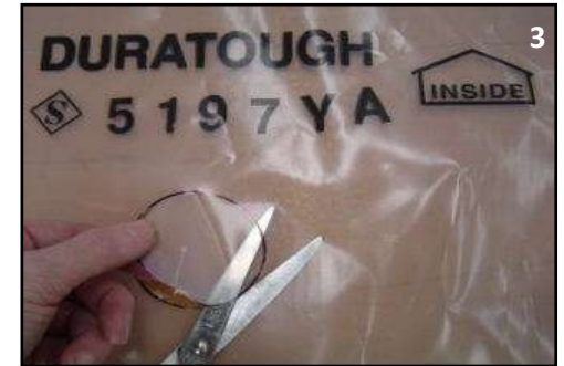
Cut out the 60mm hole, taking care not to accidentally cut the outer twinskin cover.
