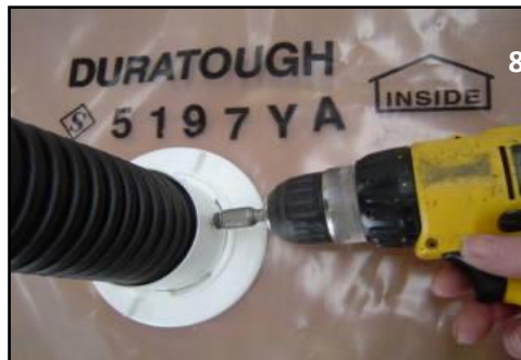
Position a Tek screw to secure all of the parts together in case of high wind load
